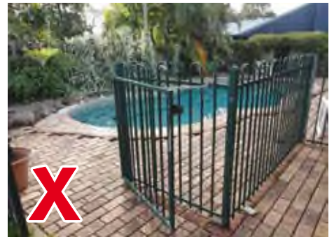
A gate cannot be tied or propped open when not in use and must self-close from any position.
