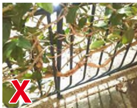
Vegetation that can be used to climb into the pool area should be removed.
