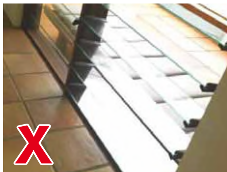
Louvres that create a gap of more than 100 millimetres do not comply.
