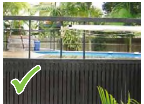
This deck bracing has been covered up with vertical palings less than 10 millimetres apart.
