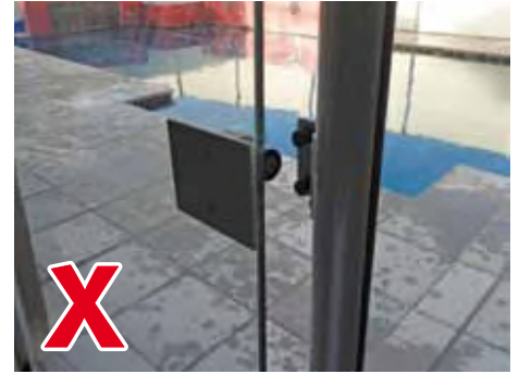
The gate or components may need to be adjusted or replaced to ensure the self-closing mechanism works properly.
